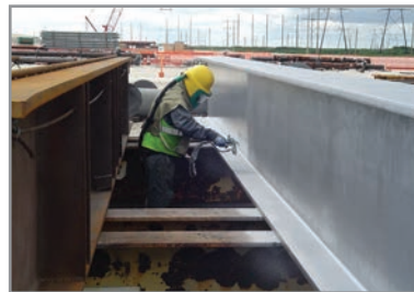
Rust Grip® application on Zachry Cranes, Houston, Texas
